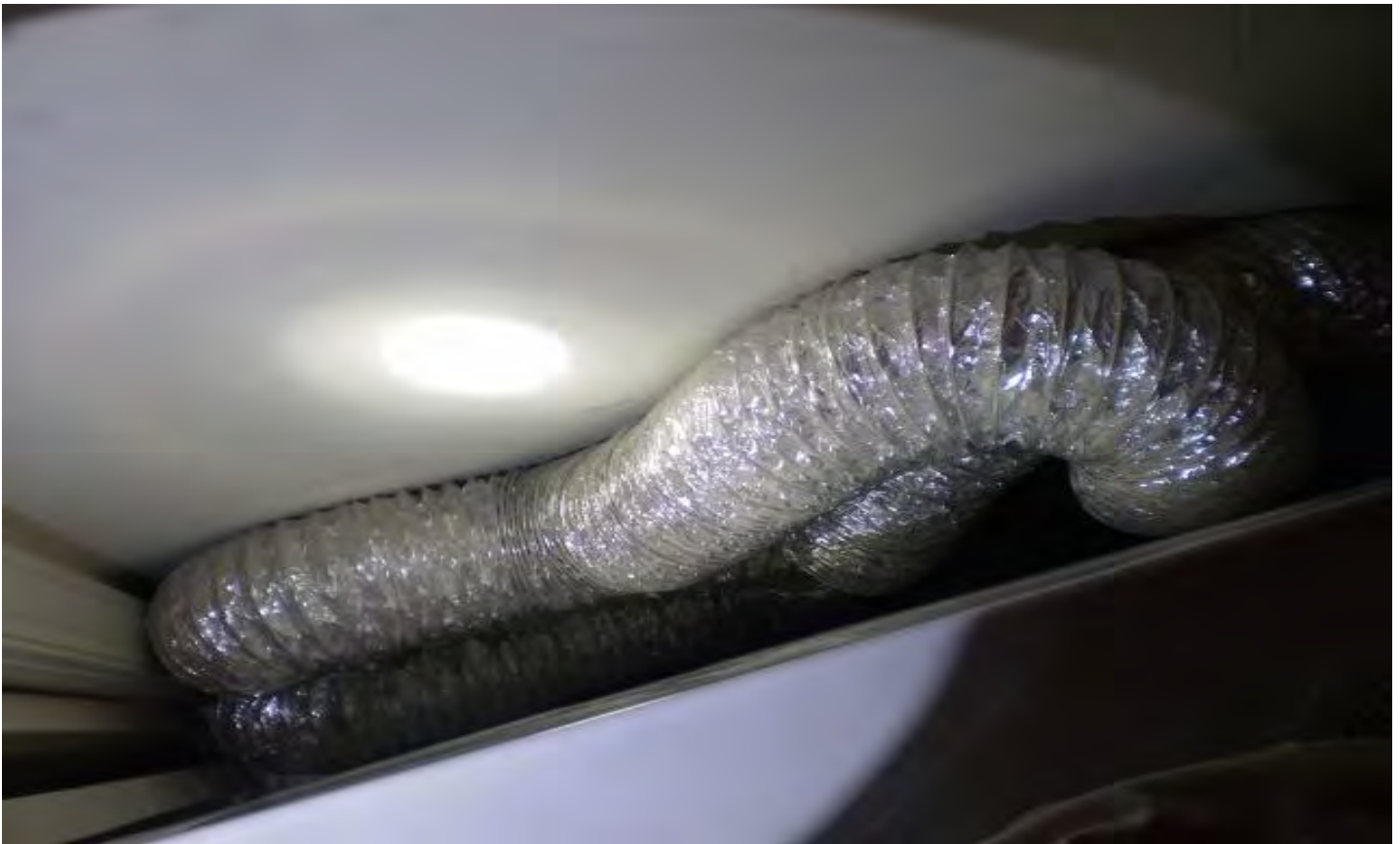
Photo # 6 View of the over-length coiled clothes dryer vent hose that should be reduced.
